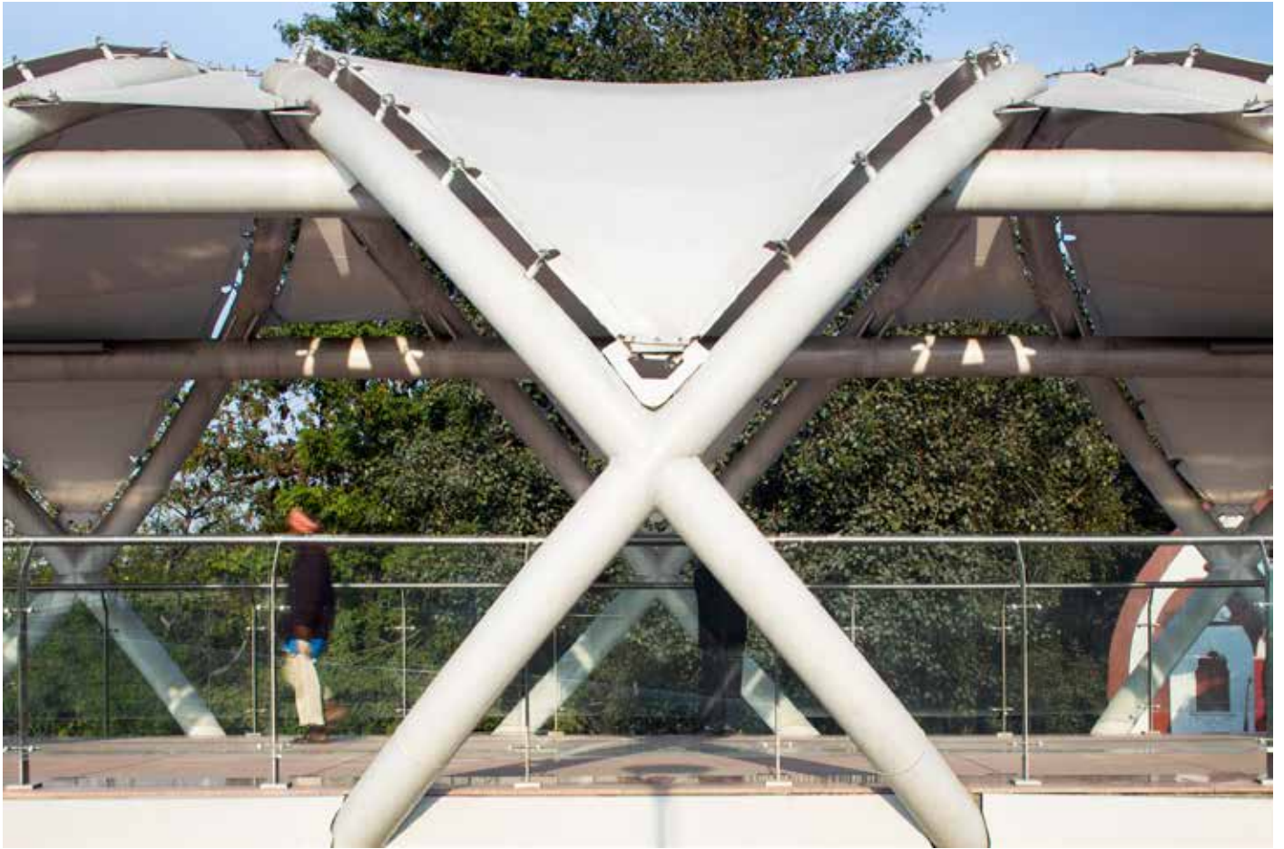
52 The criss-cross boot lace trusses are covered with tensile fabrics, resulting in the unique silhouette of the skywalk.
