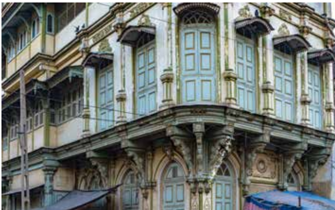
The other face becomes clearer, and you can notice it being present on the buildings themselves, their age and decay starkly visible if you took a closer look.
