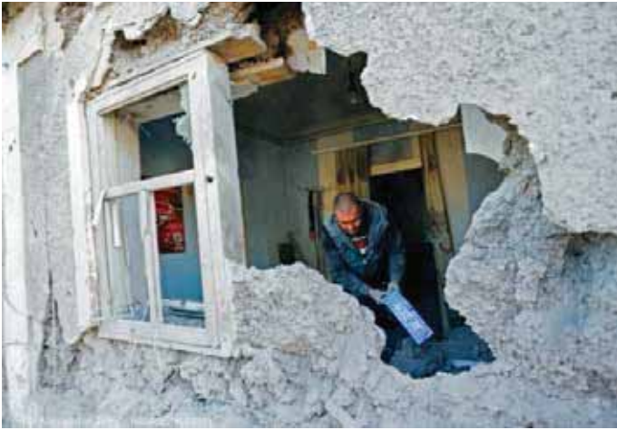
Fig.2: Damage to a residential building (Source: Retrieved, January 15,2023 from https://www.kyivpost.com/ )
