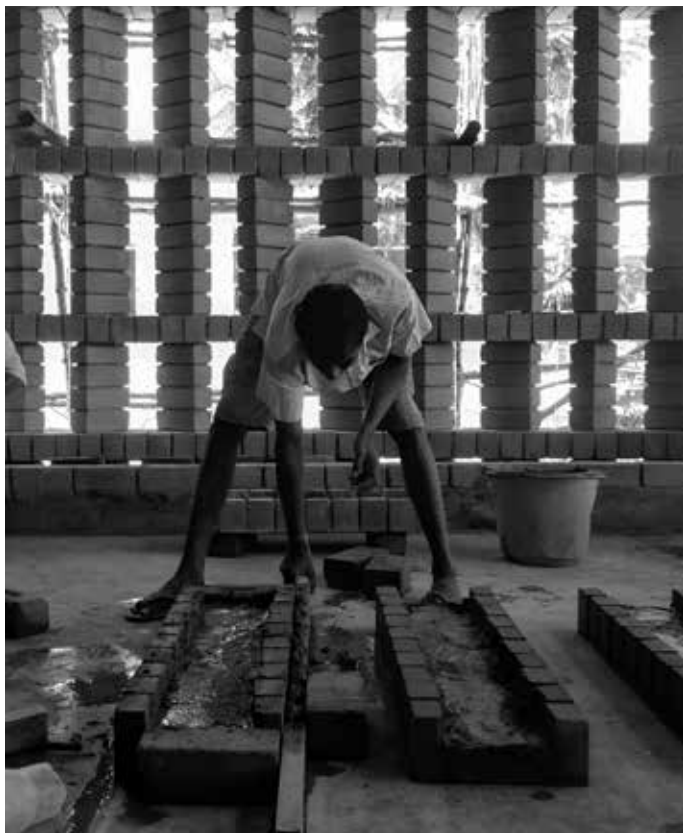
Our Mason precasting the brick beams to be used in the envelope wall.
