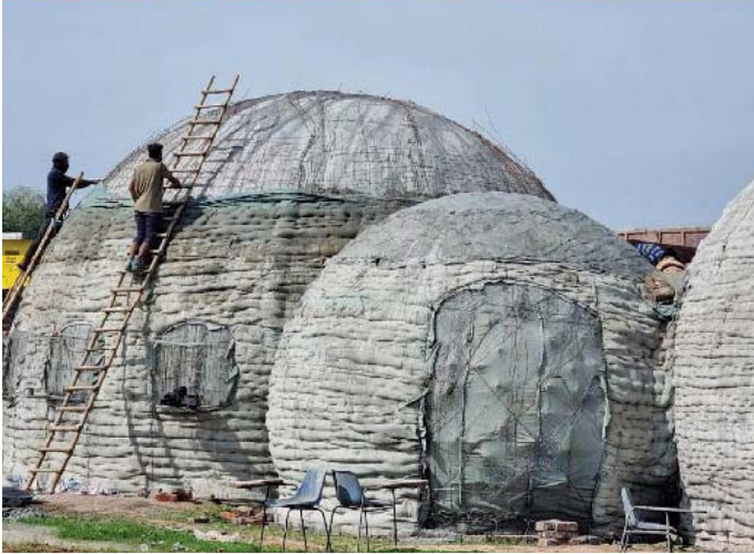
Fig. 9: An example of Radial Formwork and casting of the composite shell by Spur D Source: Author
