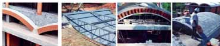
03. SEGMENTAL ARCH VAULTS - Compression roofing in low fired brick - reduced steel and cement.
