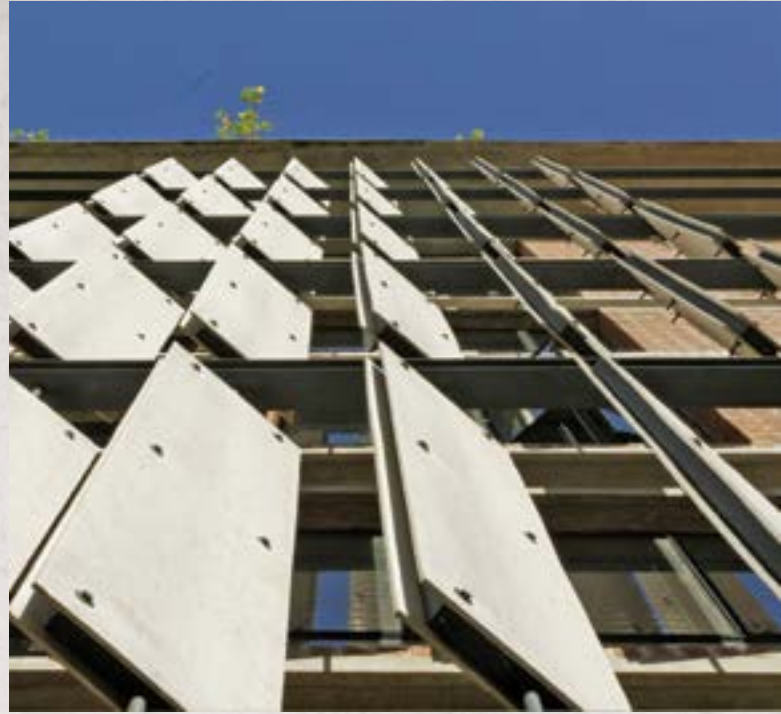
Sub Breakers Fins in the West Facade
