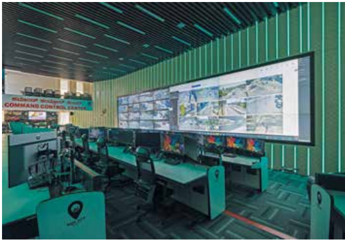
Figure 8: Command and control room
