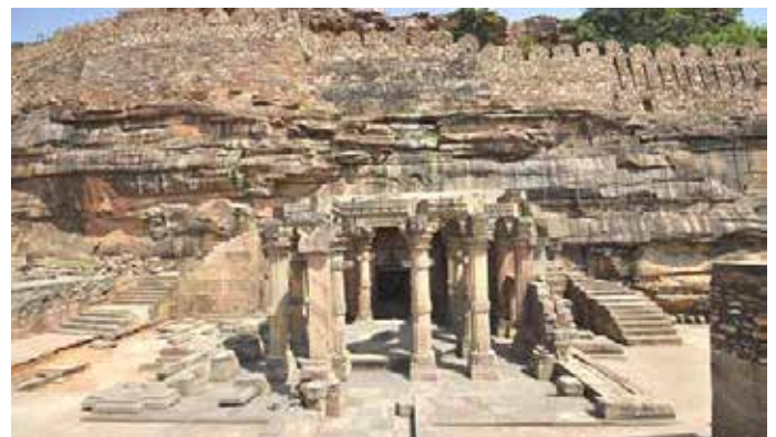
Figure 3: Neelkanth temple's mandapam in dilapidated condition Source: https://banda.nic.in/gallery/kalinjar-fort/
