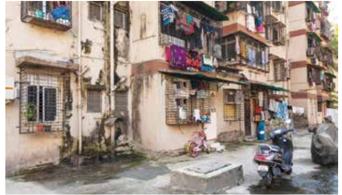
Figure 4: Common downtake pipe Source: Author
